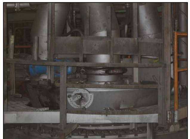
Classifier Outlet Pipes
